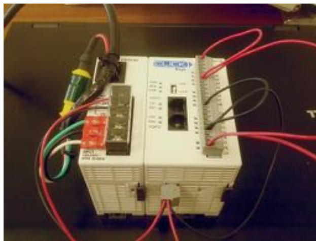
Figure 22.4: Prototype CLICK PLC for the alarm system during testing at Argonne.
