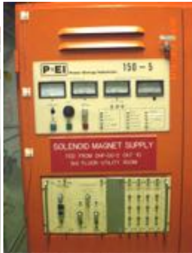
(b) Control Panel
