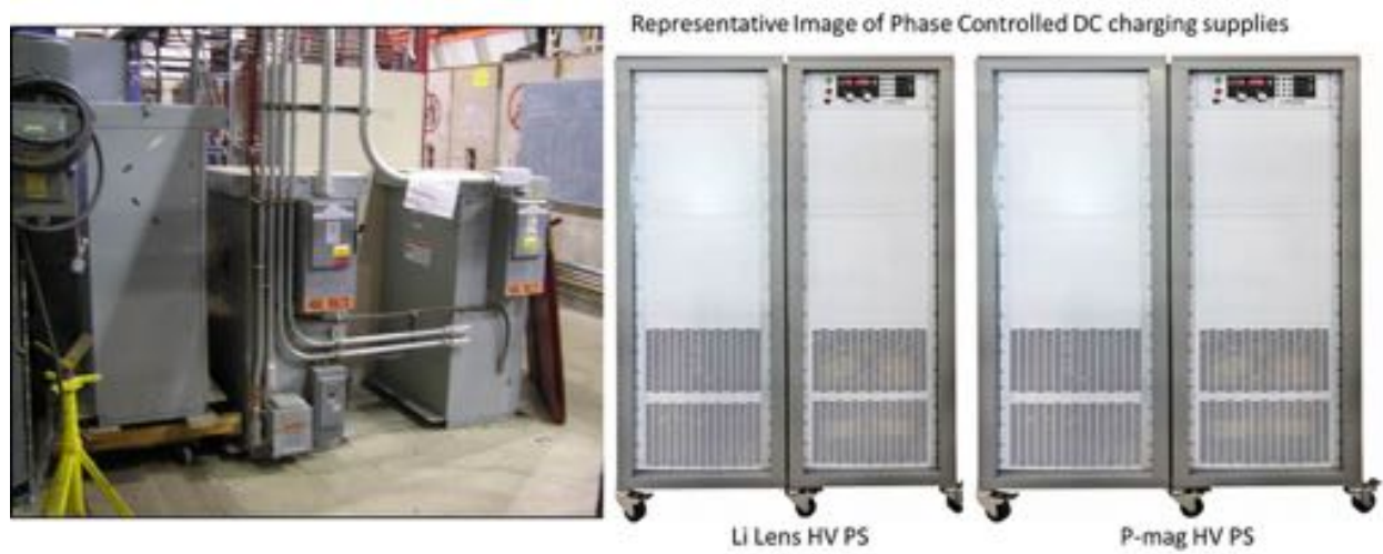
Figure 7.21: Existing 480 VAC transformers ( left ) that will be replaced by new phase controlled DC charging supplies ( right ).
