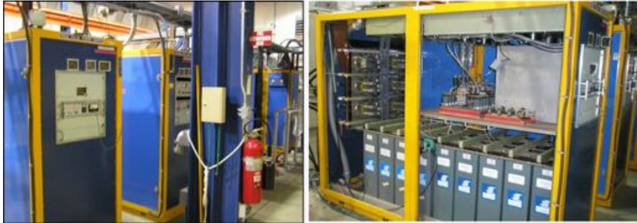
Figure 7.19: Existing lens and PMAG power supplies at AP0.
