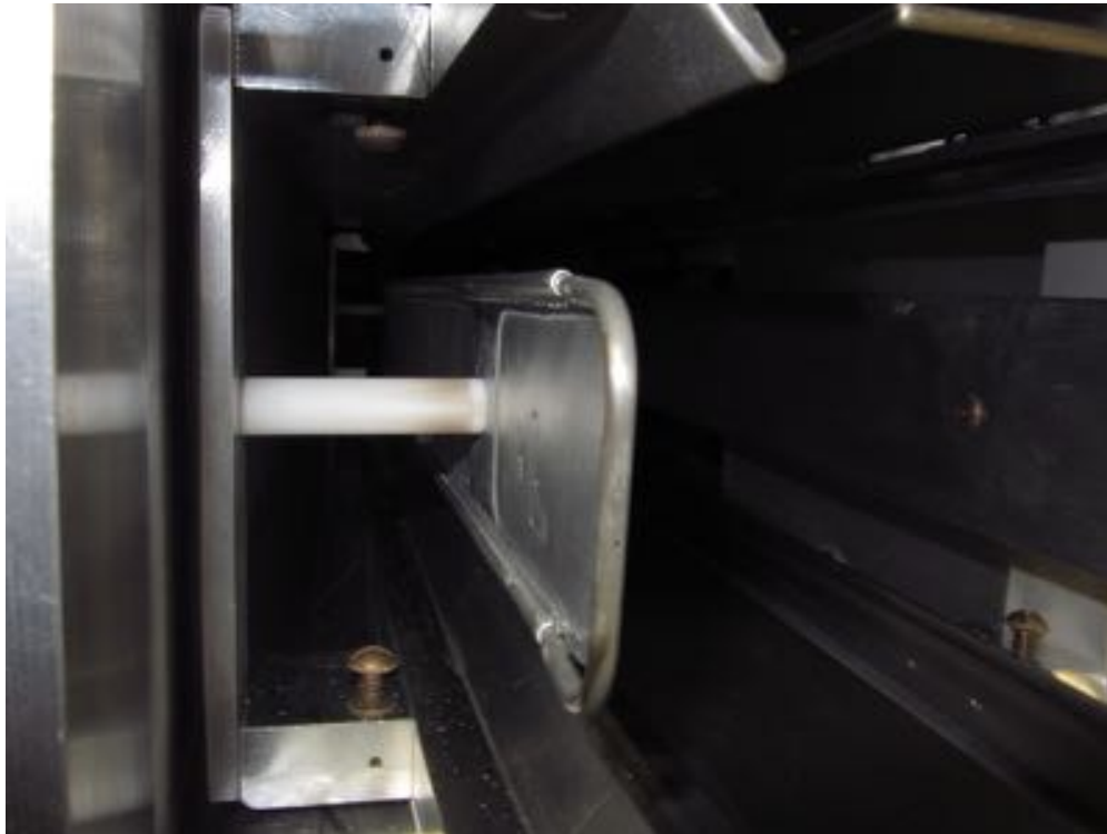
Figure 13.14: The side support insulators are varnished due to trapped electron obstruction during negative muon operations at BNL (darkened appearance close to the plate).
