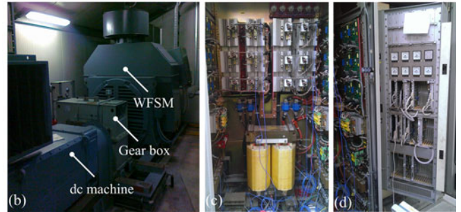
Fig. 2. (a) Block scheme of the experimental equipment (single three-phase LCI-fed WFSM if switch B is open and switches S are in the upper position, dual three-phase LCI-fed WFSM with independent converters if switch B is closed and switches S are in the upper position, dual three-phase LCI-fed WFSM with interconnected dc links if switch B is closed and switches S are in the lower position); (b) dual three-phase machine used as the LCI-fed motor and dc generator used as the load; (c) converter and input transformer cubicle; and (d) control cubicle.
