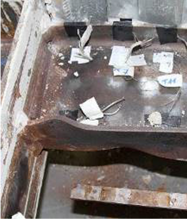
Fig. 6. Failure configuration for the full-scale specimen due to local buckling.
