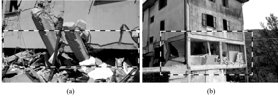
Figure 12 (a) Ejection of the infills (Arquata del Tronto) and (b) soft storey mechanism (Amatrice)
