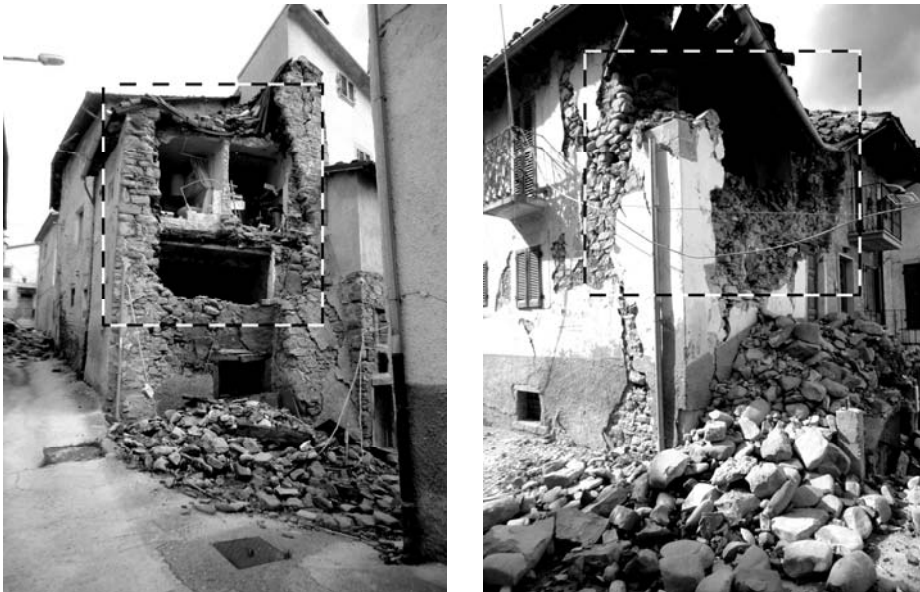
Figure 10 Out-of-plane overturning of the perimeter wall (Accumoli)
