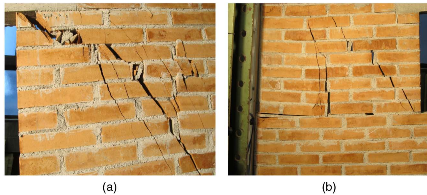
Fig. 17. Final damage pattern in the right side panel: (a) right of the opening; (b) left of the opening
