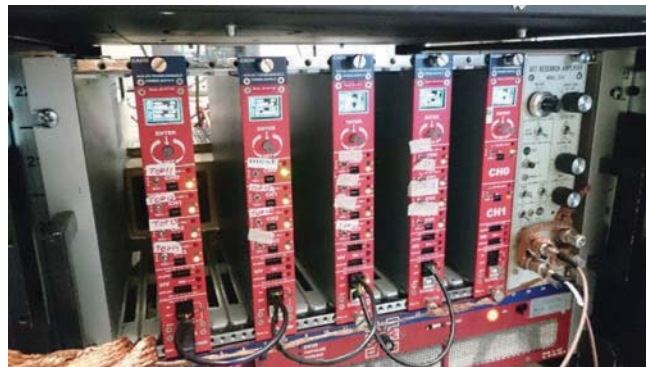
FIGURE 6.34: CAEN HV PSs used for automatic control over HV to be implemented
