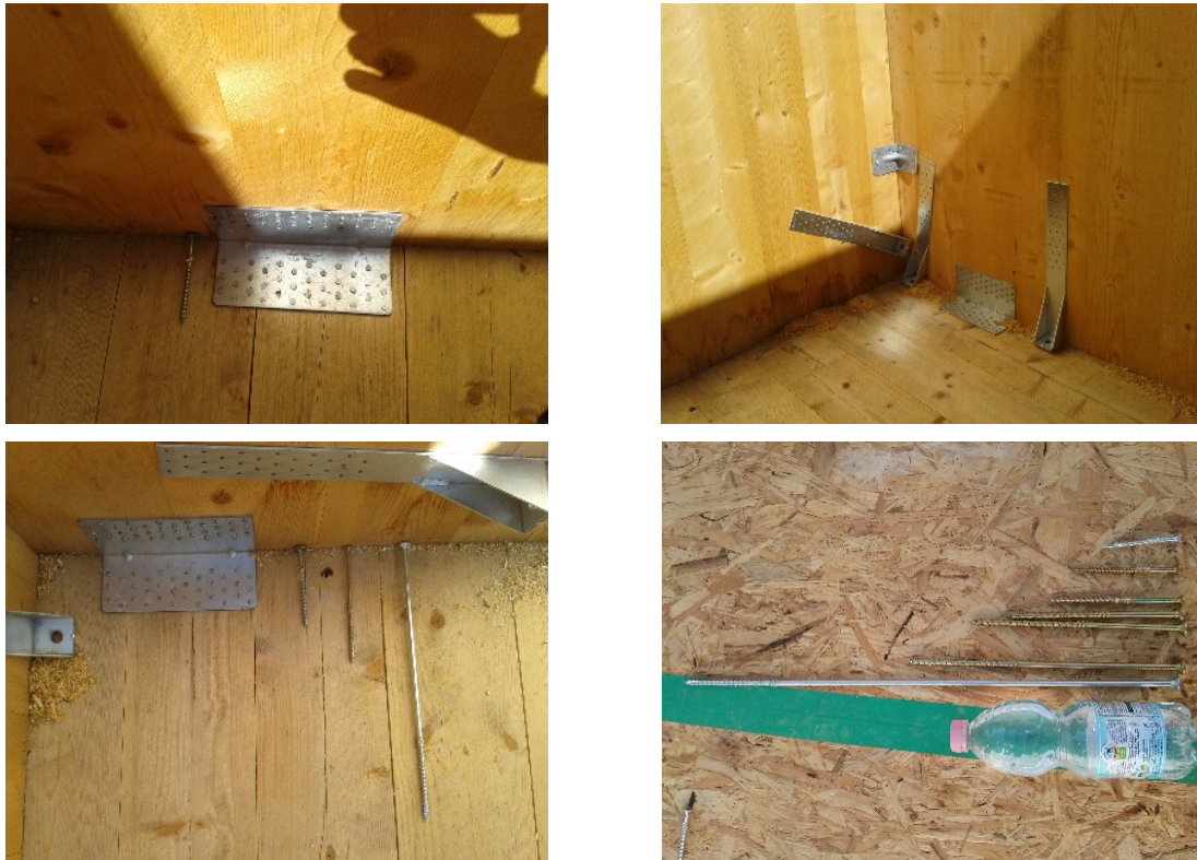
Figure 2 – different types of screws, joints and junctions used with precast timber panels. Pictures from different building constructions
