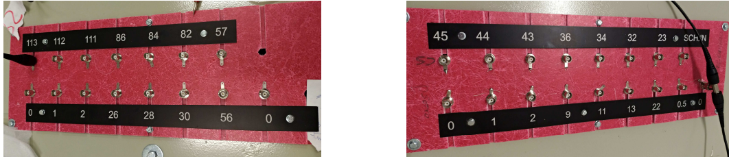
Figure 100 – Detail of the primary HV (left) and secondary LV (right) terminal block
