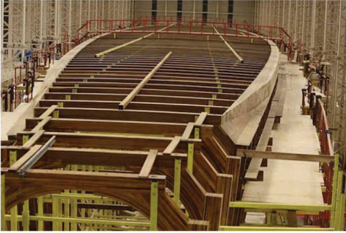
Figure 1. The construction of the Dream Symphony hull made of Iroko glued laminated timber [from www.dsv-projects.com].
