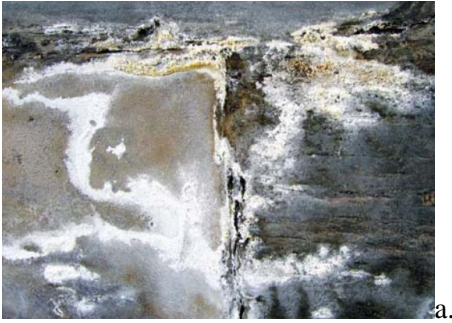
Figure 1.3 Formation of salts forming efflorescence on the surface of sandstone masonry, focused at joints between masonry blocks. [28].
