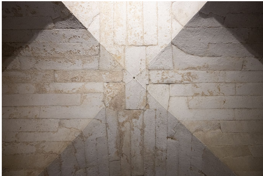
Fig.9 Groin vault in the lower chamber of the Mausoleum of Theodoric in Ravenna
