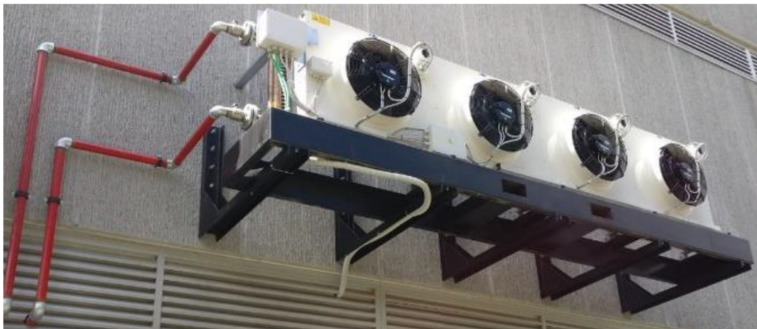
Figure 75. Fuel cell dry cooler installed in the test rig. Photo by the author.
