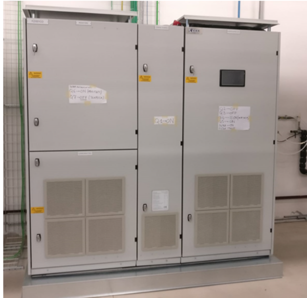
Figure 101. Power converter installed in the test rig. Photo by the author.
