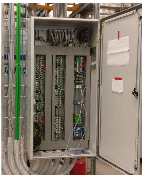
Figure 120. Test rig automation cabinet with compactRIO controller. Photo by the author.
