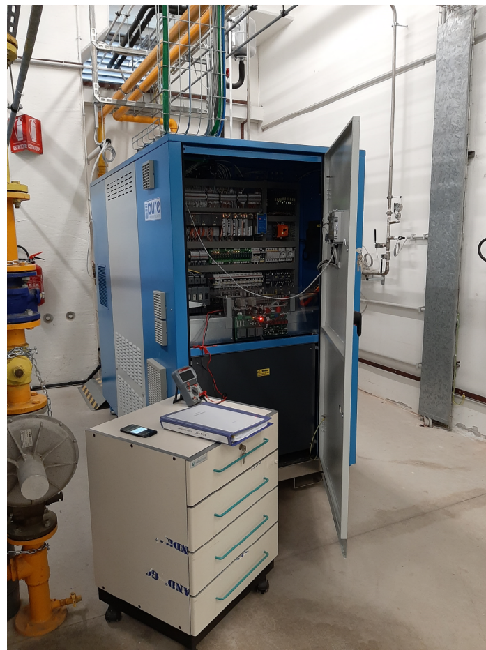
Figure 130. electrolyser during the experimental characterization tests. Photo by the author
