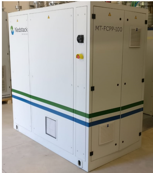
Figure 68. Fuel cell generator in the test rig. Photo by the author.
