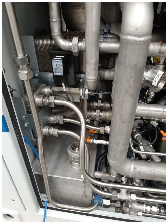
Figure 150. Fuel cell generator. Internal water tank (bottom left). Photo by the author.
