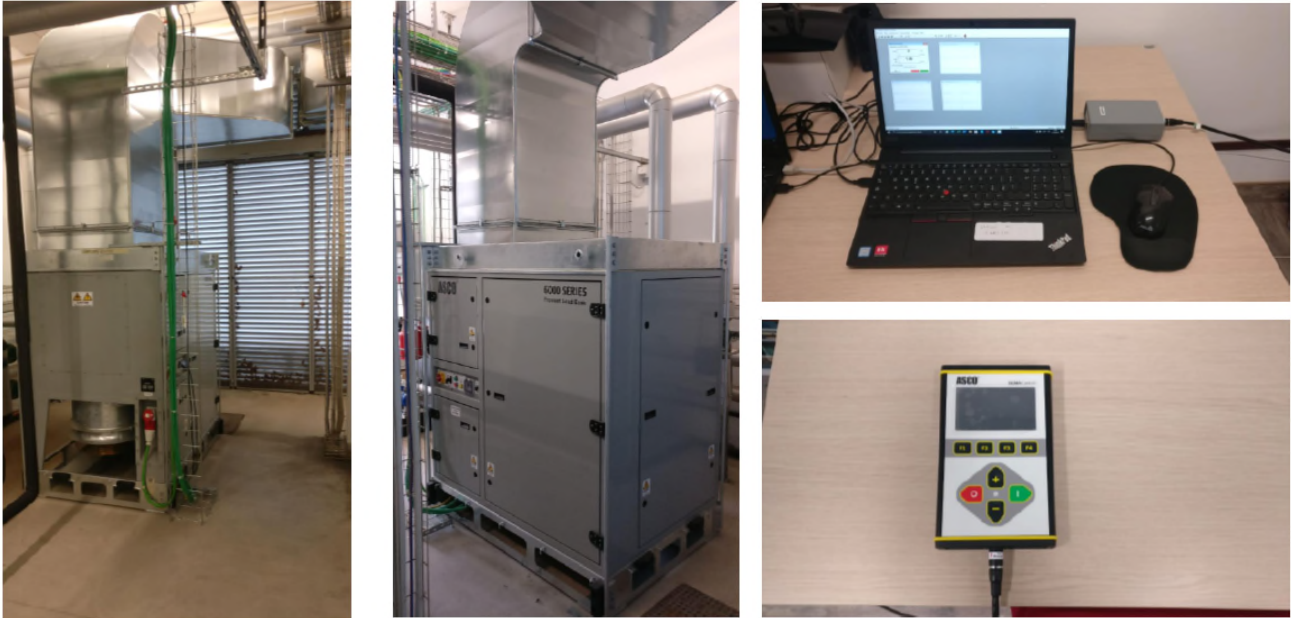
Figure 114. The load bank installed in the test rig (left). Hand-held and software-based control systems (right). [94]
