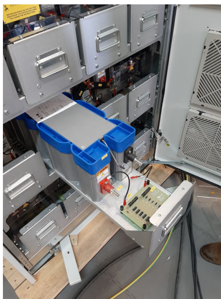
Figure 102. Power converter supercapacitors. Photo by the author.
