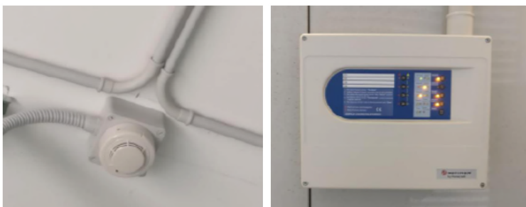
Figure 116. Test rig. Fire detection system. [94]
