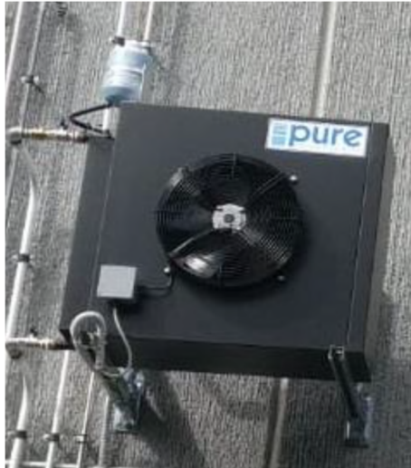
Figure 60. Pure H2-5 Alkaline Electrolyser dry cooler. Photo by the author.
