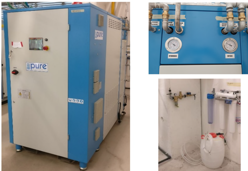
Figure 59. Alkaline Electrolyser and water treatment. Photo by the author.
