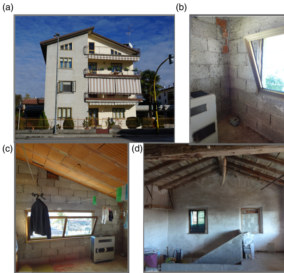
Figure 3. (a) An example of a three-story masonry building belonging to the considered typology and the details of (b) blocks constituting the load-bearing vertical structure, (c) rigid roof, and (d) pre-existent wooden roof. The color version of this figure is available only in the electronic edition.
