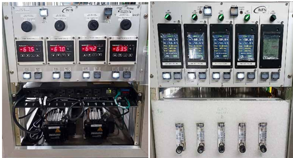
Figure 3.14: Humidity monitoring system installed in E-hut.
