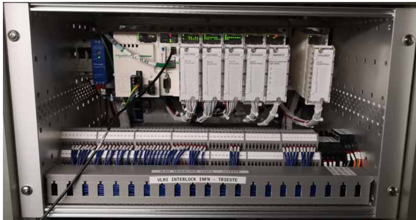
Figure 3.15: VLHI PLC installed in E-hut.
