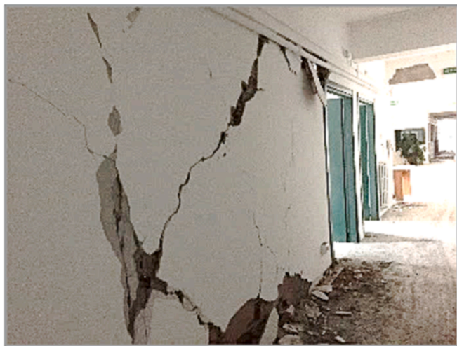
Fig. 16. Image of Lo2-type partition panel situated in the C/6-C/7 span on ground storey taken after 30th October 2016 earthquake.
