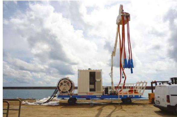
Fig. 4. Mobile structure for ships' cold ironing in the port of Genoa (Source: Port System Authority of the Western Ligurian Sea)
