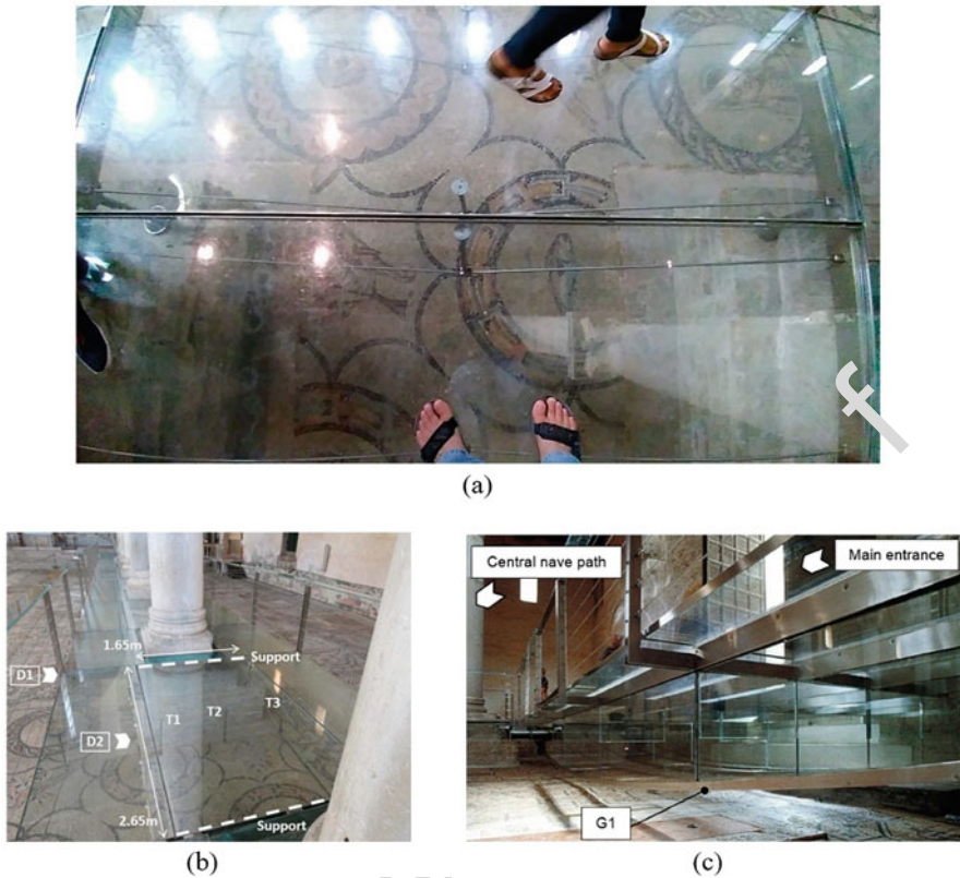
Fig. 13.2 Vibration analysis of an existing in-service glass walkway: (a) visual inspection and (b–c) details of the structural system. (Figures reproduced from [9] under the terms and conditions of the Creative Commons Attribution (CC BY) license)
