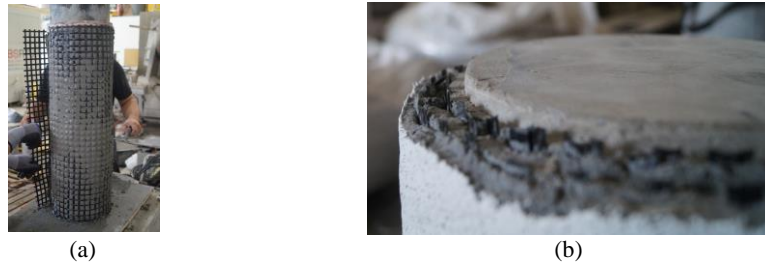
Fig. 1 Retrofitting of a column with B-TRC (a) and detail of a B-F/TRC retrofitted column (b).
