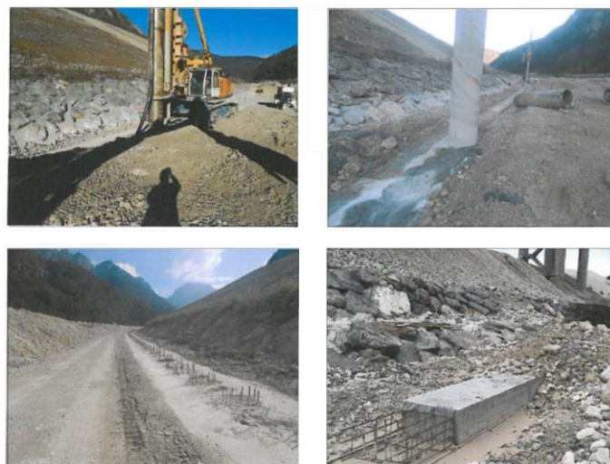
Figure 18 - Realization of the external barrier at the foot of the tailings dams (Protec, 2017).
