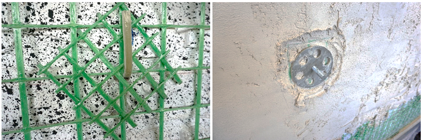
Fig. 2. View of the connectors during construction: (a) L-shaped GFRP connectors before application of coating and (b) artificial diatone during application of coating.
