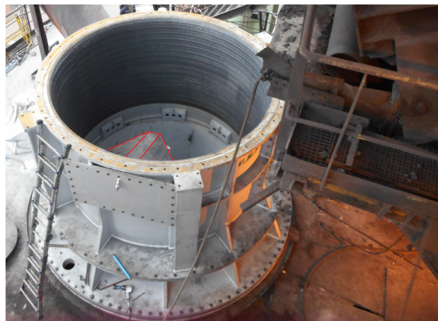
Figure 2. Photograph of the currently installed fixed hopper, where the two-skewed deflector is highlighted in red. It can be seen an external hatch on the hopper. For maintenance purposes, the deflector, attached to the hatch, can be easily removed.
