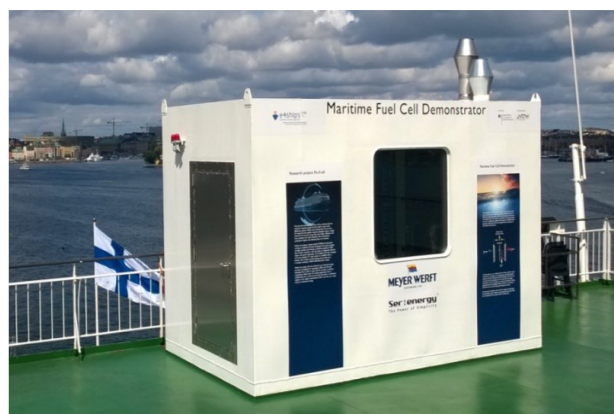
Figure 86 - Prefabricated HT-PEM fuel cell module onboard MS Mariella [244]
