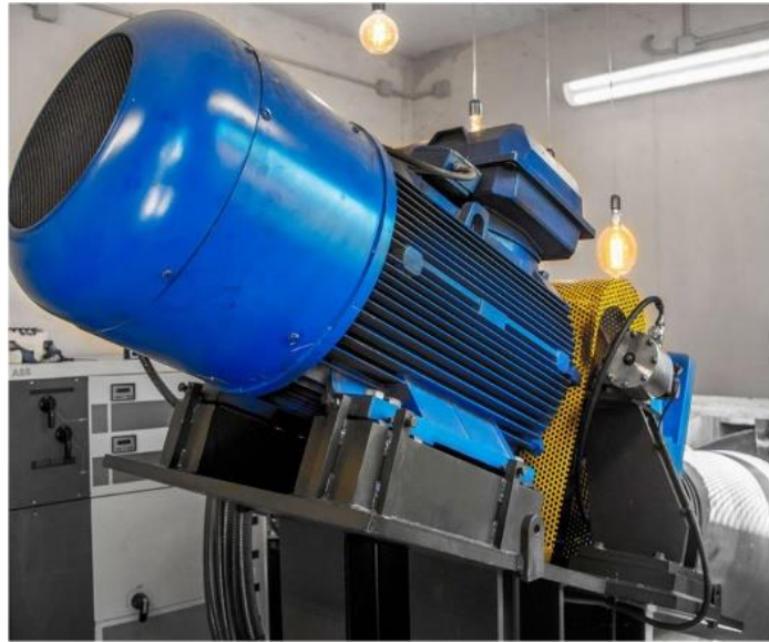
Figure 6: Example of an electric generator coupled to a skew turbine for a hydropower group.
