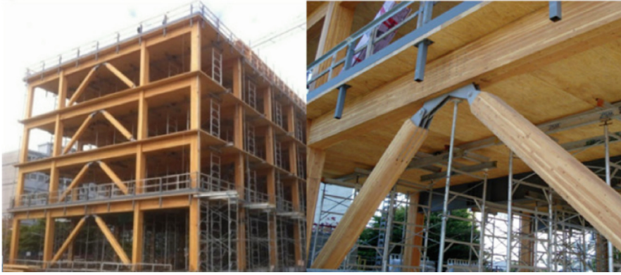
Fig. 1. Example of timber structure. Figure reproduced from [6] under the terms and conditions of a CC-BY license agreement.
