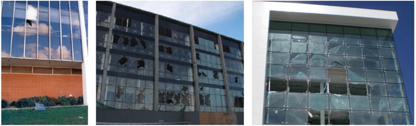
FIGURE 1 | Examples of structural damage observed in real glass facades after earthquakes. Figures reproduced from [4] with permission from Elsevier©, license number 6110680457389 (September 2025).
