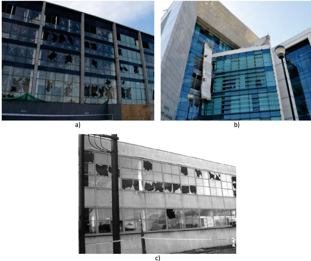
Figure A.2-1 (a) Glazing damage in Chile, after the 8.8 Chile Earthquake (2010) (FEMA E-74_Figure 6.3.1.4-3); (b) Impact damaged façade at the entrance of the Corte de Apelaciones de Talca , after the 8.8 Chile Earthquake (2010) (FEMA E-74_Figure 6.3.6.1-2); (c) Damaged glazing system in San Francisco (1989), after Loma Prieta earthquake
