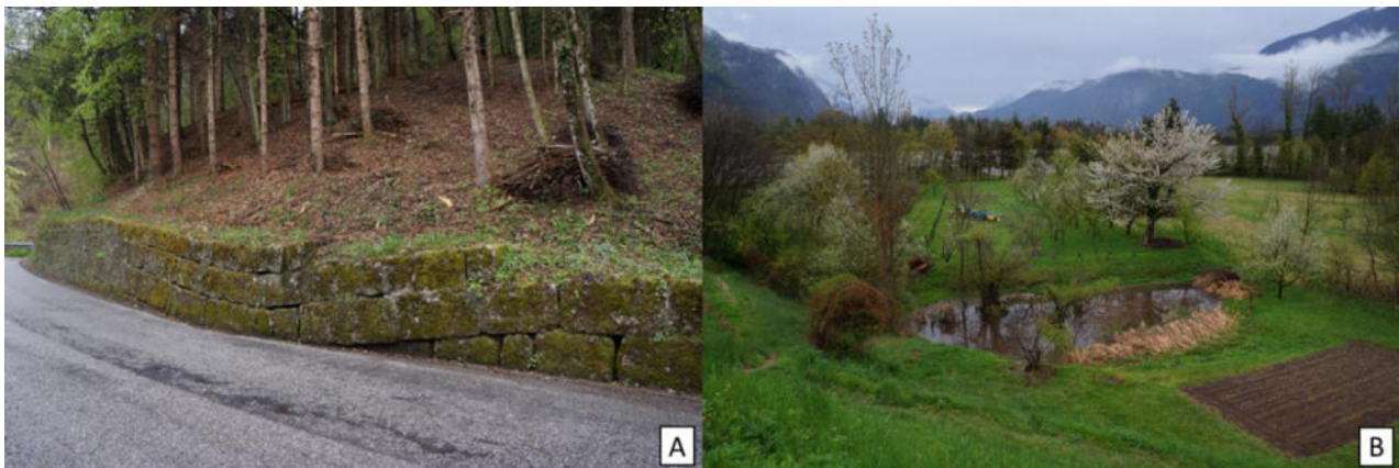
Figure 55 A) Deformed retaining stone wall; B) Depression artificially filled with water located North of the sinkhole (photo taken from NW)
