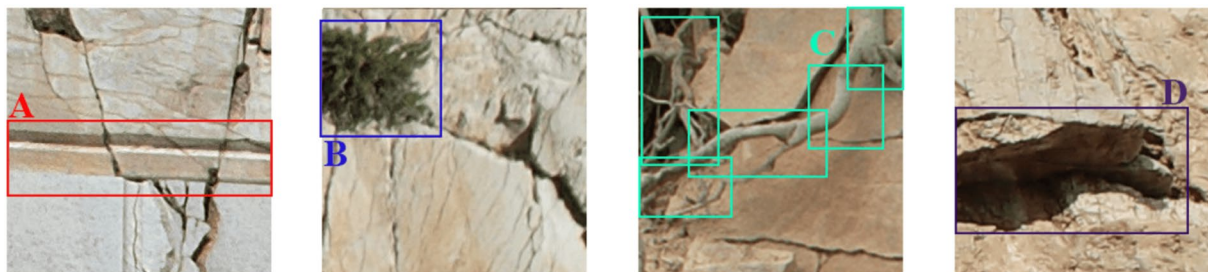
Fig. 2 Common scene artifacts: (A) Blast holes. Occlusions due to (B) vegetation and (C) roots. (D) Shadow effects.
