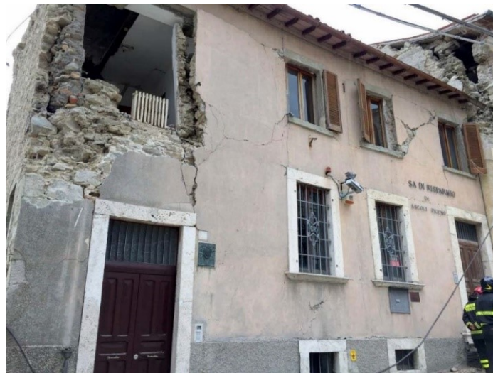
Figure 4 Damage on a URM structure after the Central Italy earthquake (2016): localised in-plane shear damage in the masonry piers of the upper floor and out-of-plane expulsion of the left-corner wall (Da Porto et al., 2016)
