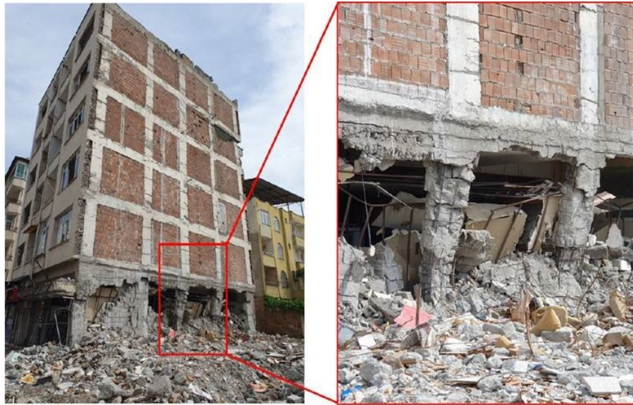
Figure 23 Soft-story mechanism in a masonry-infilled reinforced concrete building – Syria and Turkey earthquake, 2023 (ReLUIS and Eucentre, 2023)
