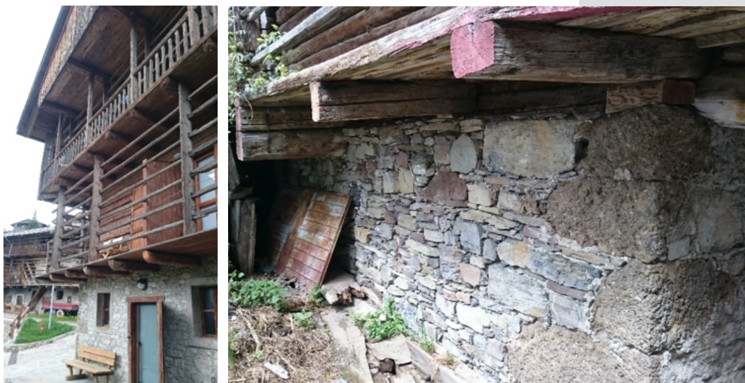
Figure 4. (a.) Sight of the main facade of a three-storey Sauris house. (b.) Load-bearing structure in stone and pebbles in a Sauris di Sopra house. At corners, the use of huge squared stones (tof) is highlighted. Authors' pictures.
