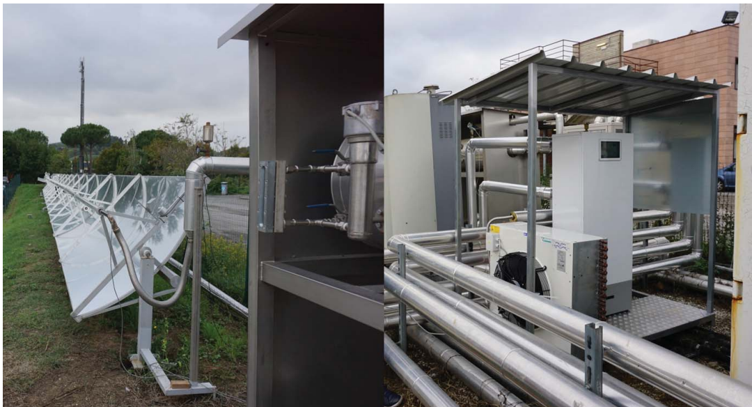
Figure 4.19: solar-ORC: left solar collector and tracking system, right ORC prototype and the dry cooling unit.
