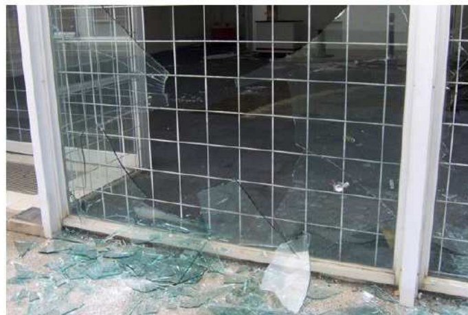
Fig. 11. Bomb blast net curtain: example of typical failure scenario after bombing
