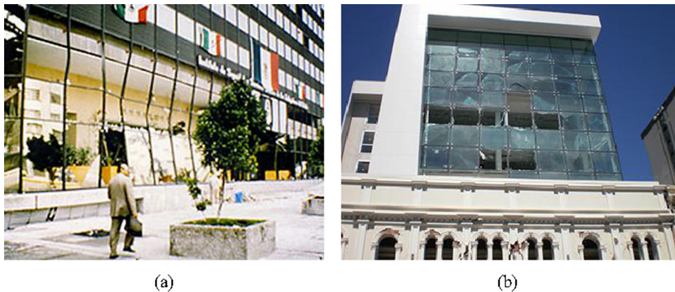
Fig. 5. Examples of damage scenarios in glass curtain walls due to seismic events: (a) Mexico City (1985) and (b) shattering of glass panes in a commercial building (photo: J Bothara).
