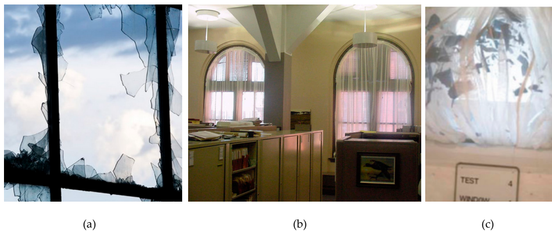
Figure 14. Glass windows and facades under shock: (a) example of severe damage of un-protected window and (b,c) enhanced performance in presence of textile curtain nets.
