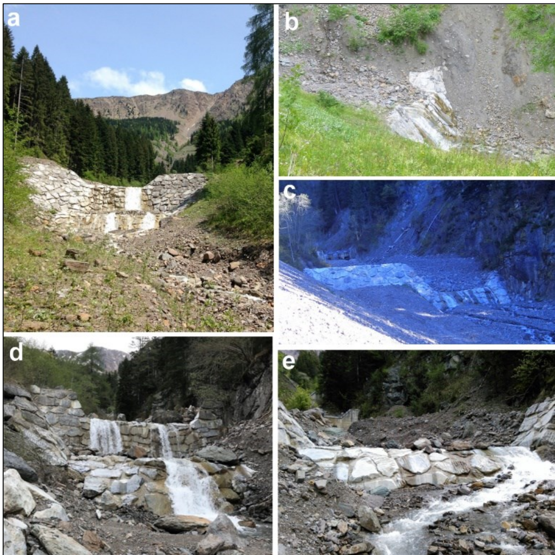
Figure 4.5: Check dams built along the Moscardo stream between 2005-2006 (Fig. 4.2). a) Check dam (n. 15) built in the lower part of the Moscardo channel. Cucchiario 2018; b) Check dam (n. 25) built in the middle part of the Moscardo channel. Cucchiario 2018; c) Check dam (n. 16) built in the lower part of the Moscardo channel. Cavalli 2006; d)
