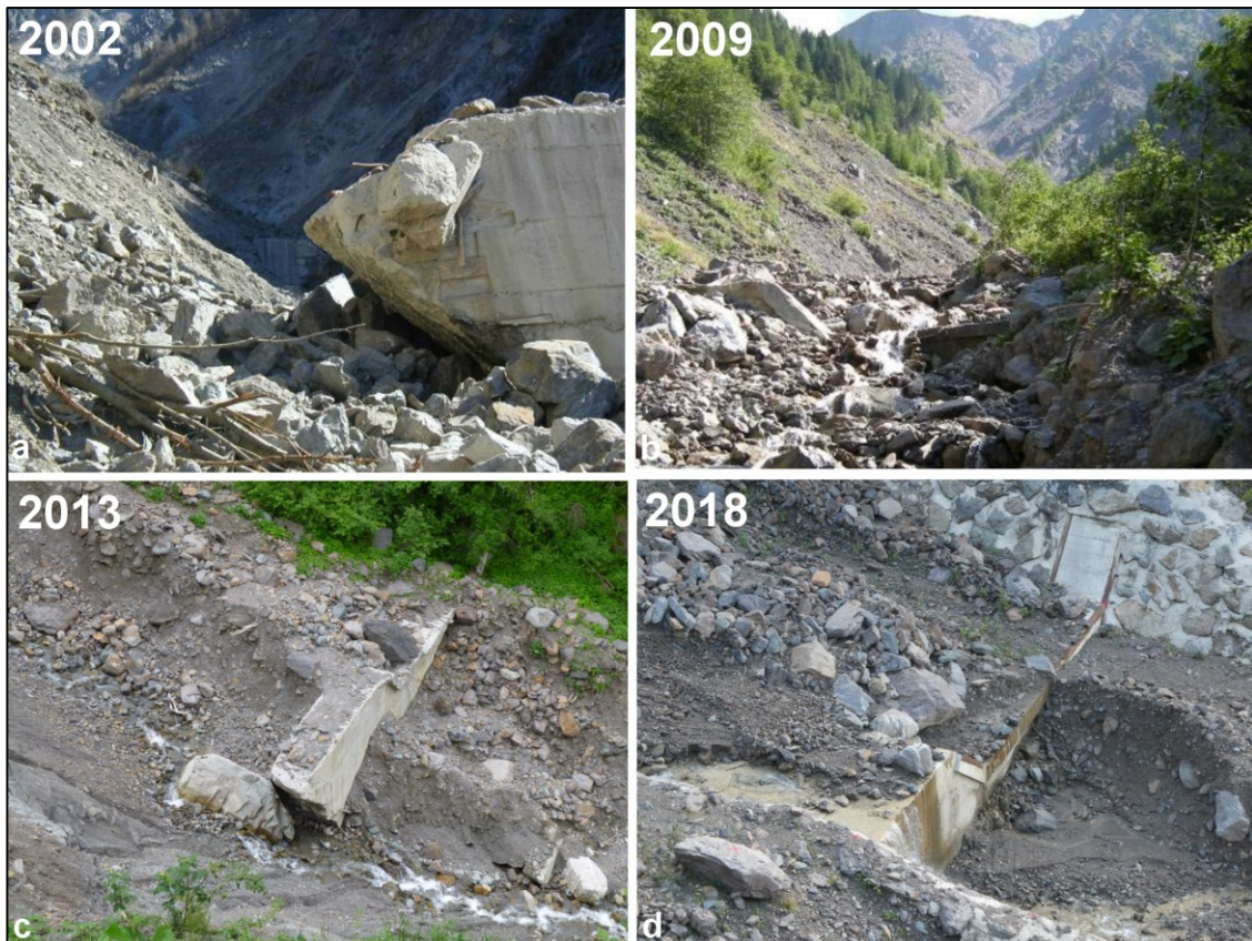
Figure 4.35: The check dam (n. 30) over time. a) The damaged right wing of the check dam in 2002 (Dini, 2011). b) The filled check dam in 2009 (Dini, 2011). c) The flanking around the check dam in 2013. Blasone 2013. d) The check dam in October 2018. The water flows on the right wing. Marchi 2018.
