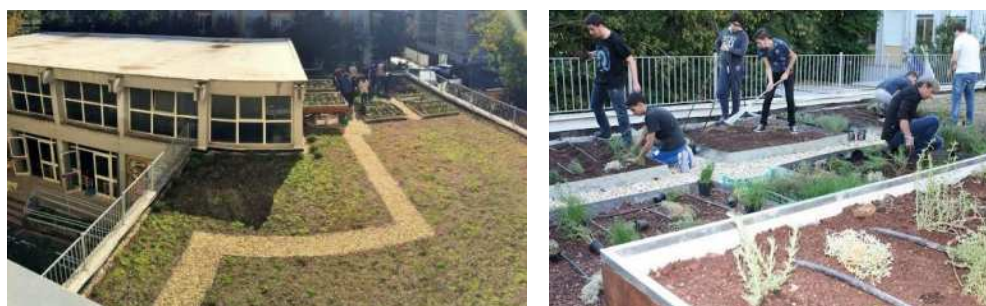
Fig.1. Experimental green roof. [a] General view, [b] installation made with the collaboration of the students
