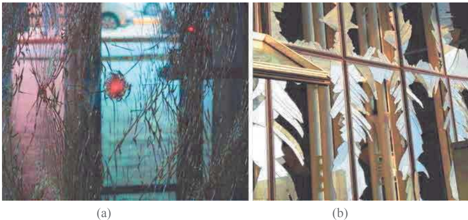
Fig. 3.2 Examples of damaged glass facades after the tragic attacks at (a) Istanbul and (b) Brussels airports
