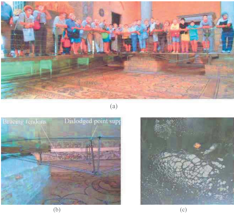
Fig. 3.5 Case-study glass footbridge: (a) live loads; (b) steel tendon and (c) local delamination
