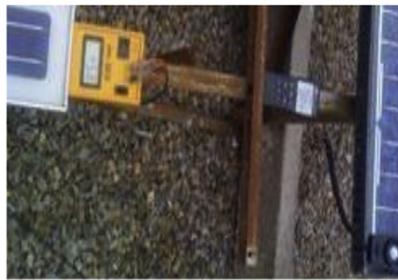
g) Reference solar cell and module temperature sensors
