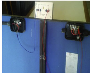
e) Connection fault ( R = 5\Omega )
