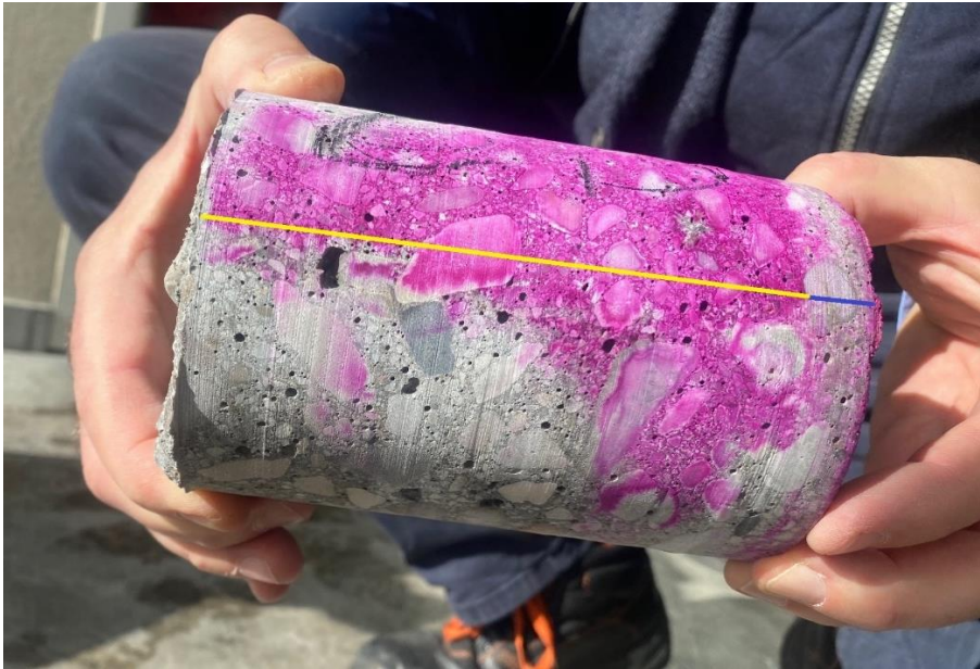
Fig. 18. Result obtained by spraying phenolphthalein on the specimen cut in Fig. 17.
