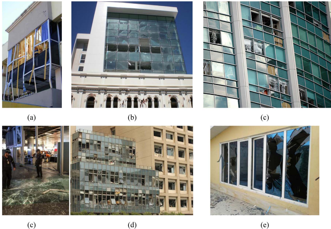
Fig. 2. Examples of glass systems under hazards: (a)–(b) seismic events, (c) hurricanes and (d)–(e) explosions.
