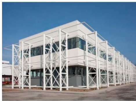
Figure 5-1: Retrofit of an existing RC building with an exoskeleton (figure reproduced from [72] under the terms and conditions of the Creative Commons Attribution (CC BY) license.
