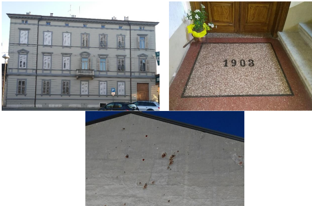
Figure 3-50: Front façade of the case study building and the construction year written at the entrance. Below, the damaged lateral façade where the clay bricks are visible.
