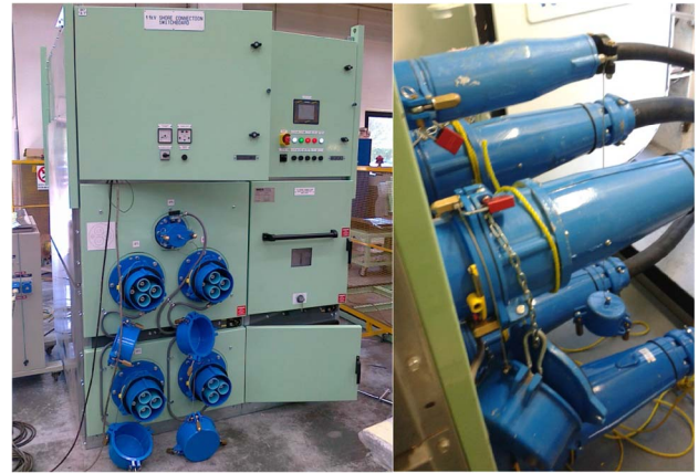
Fig. 3. Typical switchboard for shore connection purposes.
