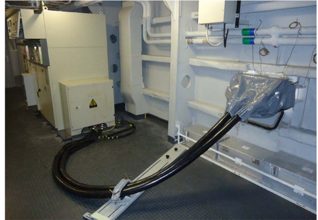
Fig. 11. Crane plugs and sockets.
