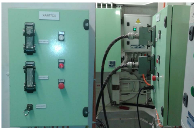
Fig. 5. Shore connection control cabinet.
