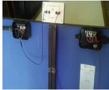
e) Connection fault ( R = 5\Omega )
