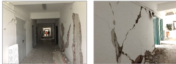
Figure 11. Images of the ground storey Lo2-type longitudinal partitions taken after 30 October 2016 earthquake
