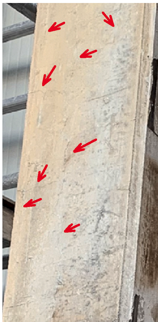
Fig. 3. Splitting cracks around reinforcements in a column in the receiving area.
