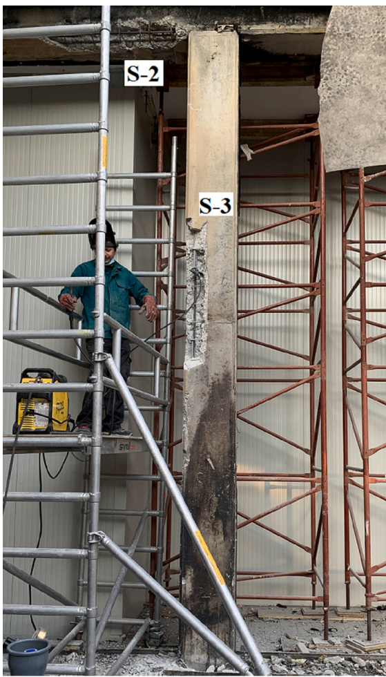
Fig. 10. Location of reinforcement samples S-2, in the beam, and S-3, in the column.
