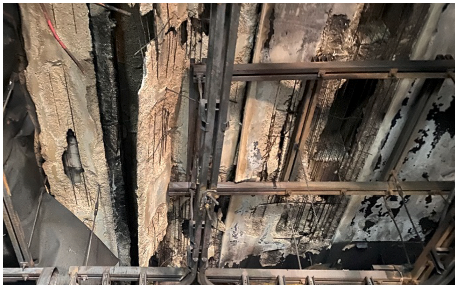
Fig. 2. Damage caused by fire in the prefabricated panels of the roof over the receiving zone.
