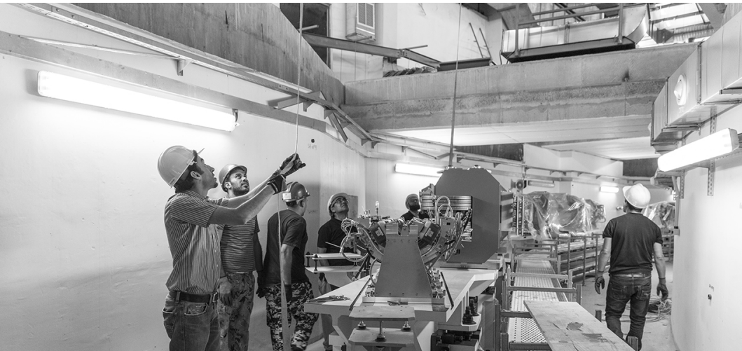
Fig. 4. Installation of a section of the vacuum chamber of the SESAME storage ring.
