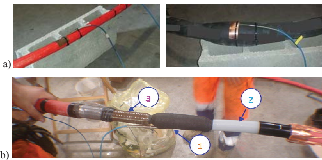
Figure 1 - View of the points of installation of the thermocouples outside the cable and the joints (mirror and main rings) a), and inside the joints (mirror ring) b).
